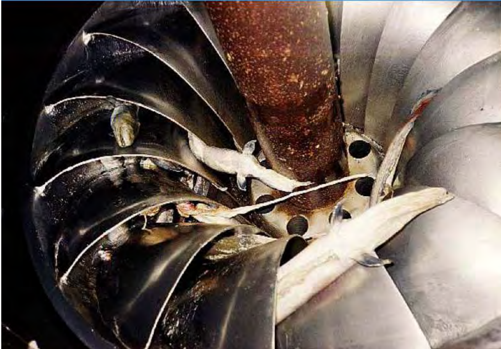
Turbine clogged with eels. Note eel skin stretched across shaft. Photo: Alex Haro, Ph.D. , S. O. Conte Anadromous Fish Restoration Center Presentation- Fish Passage in the Northeast: Old Problems, New Solutions U.S.G.S., Biological Services
